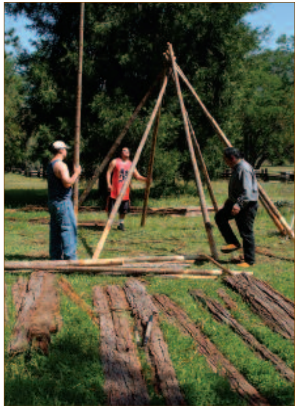
Construction of the bark house begins with a frame made of pine wood poles.
